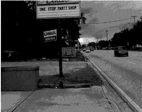
Missing sidewalk north of Vine St.
