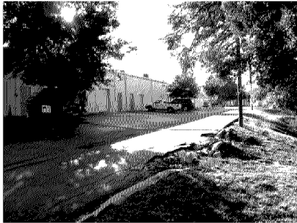
Broken curb and eroding parking lot.
